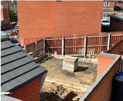
Photograph of the foundations relating to the outbuilding at No.5, taken from the rear of No.7.
